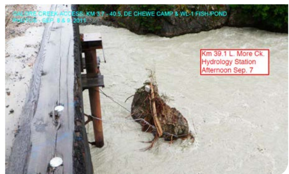
Figure 3 (top) | Flooding of access road
