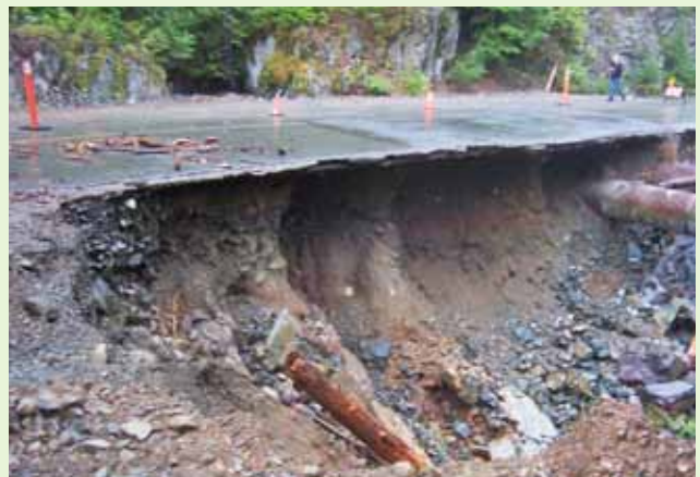
Figure 6 | Damage to main access road
